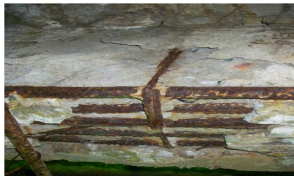
Figure 2. Damaged part of the bridge structure
